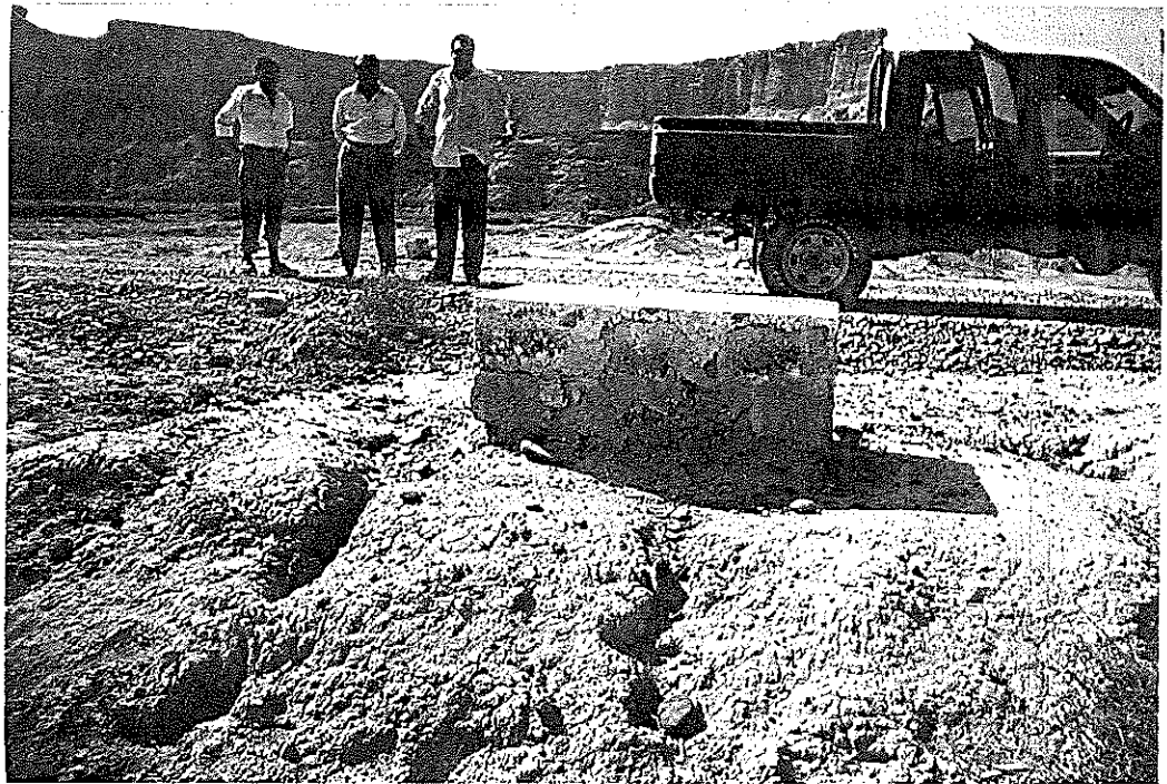
Photograph - 12 Shoulders in very bad condition at Agore - Malam Section
